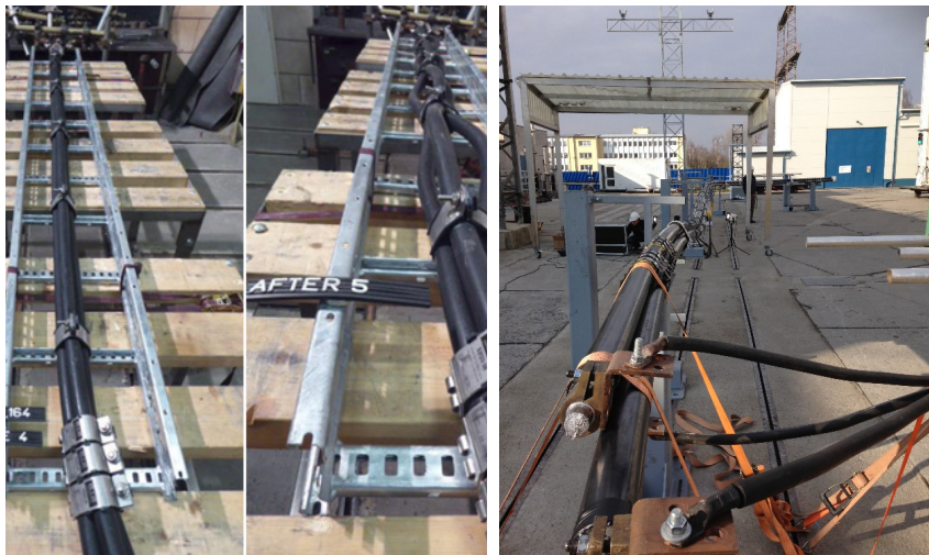
TYPICAL TESTING TO IEC 61914 AND BESPOKE TESTING OF A HV TEST RIG TO A CUSTOMER'S SPECIFICATION.
