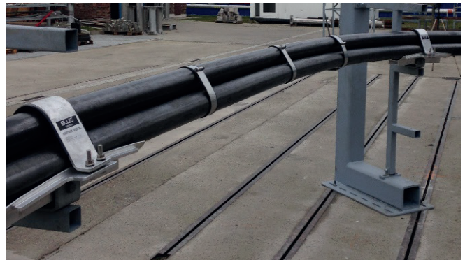
A PHOTO OF THE SHORT CIRCUIT TEST RIG FOR CENTAUR TREFOIL INCLUDING FLEXI-STRAPS. TESTING WAS CARRIED OUT AT ZKU LABORATORIES IN PRAGUE, CZ.
