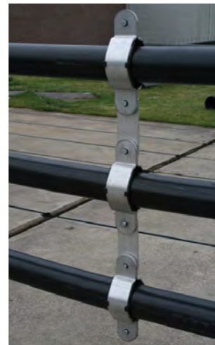
TYPICAL INSTALLATION, PHOTO TAKEN AT A SHORT CIRCUIT TESTING EVENT AT KEMA LAB, ARNHEM NL.
