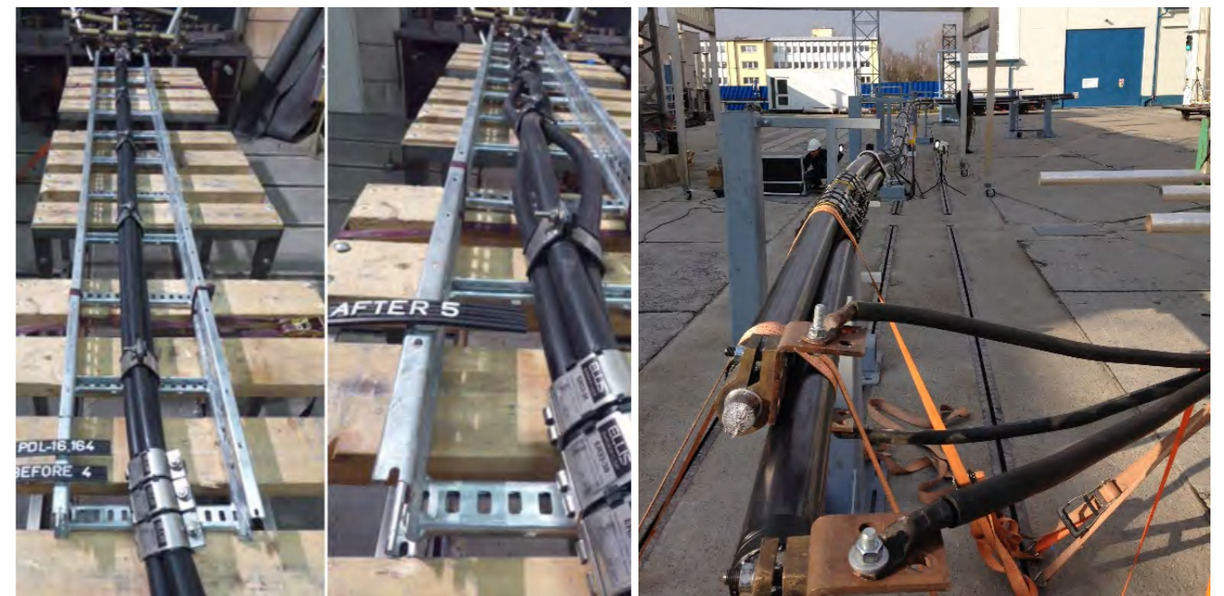
TYPICAL TESTING TO IEC 61914 AND BESPOKE TESTING OF A HV TEST RIG TO A CUSTOMER'S SPECIFICATION.
